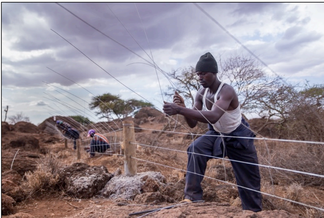
Electric exclusion fence and outriggers to keep elephants from approaching the 3 ft high fence.
